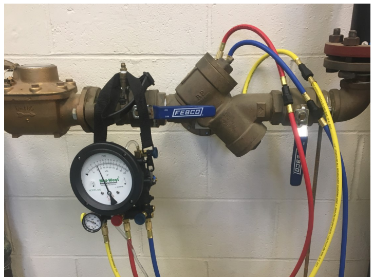
David and I tested all the backflow prevention devices located at the Main Office, Treatment Plant, Screen House, Pump Stations, and the mobile units.
